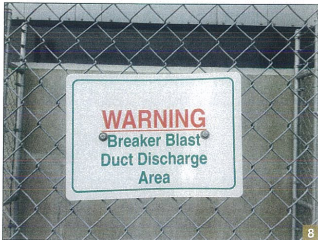
A warning for blast vents. (Used with permission from BP.)
